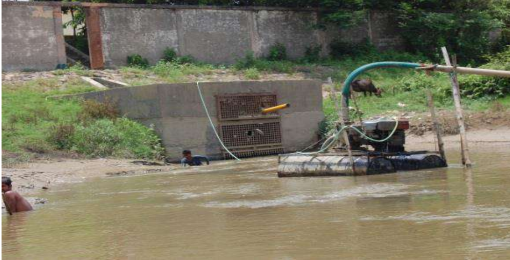
Photographs of OTC Water Intake point
